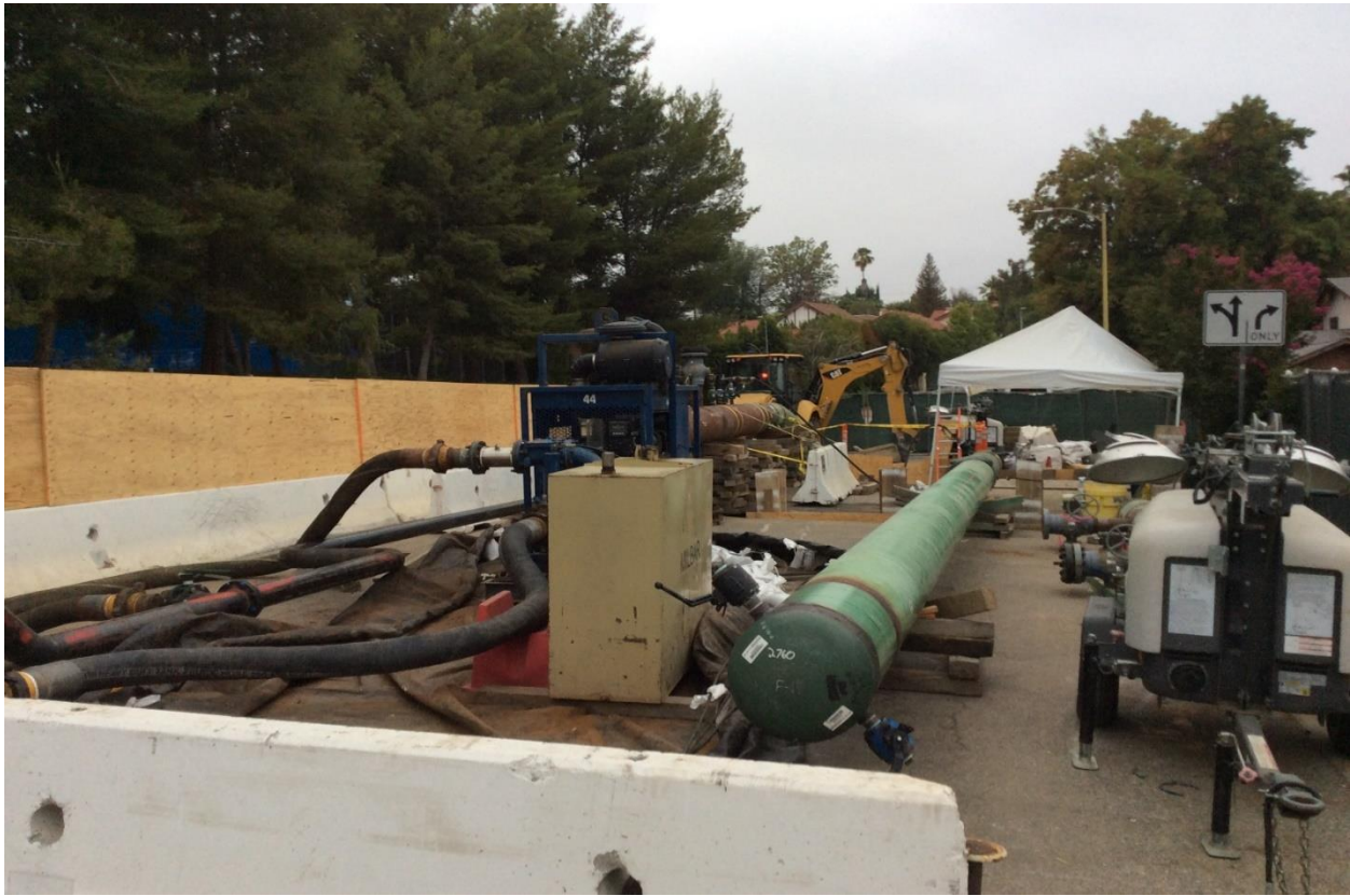
Figure 6: Pump and Test Head at Burbank Boulevard
