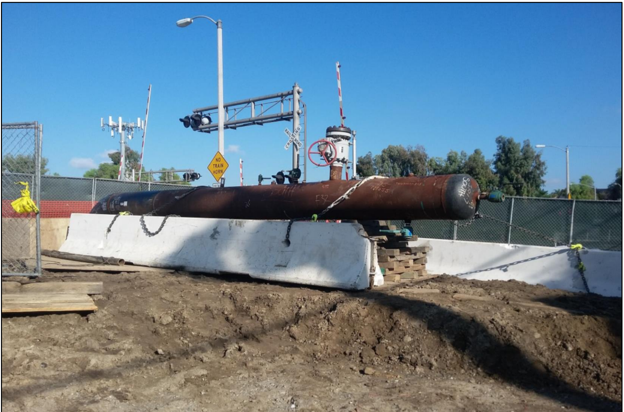
Figure 5: South End Test Head
